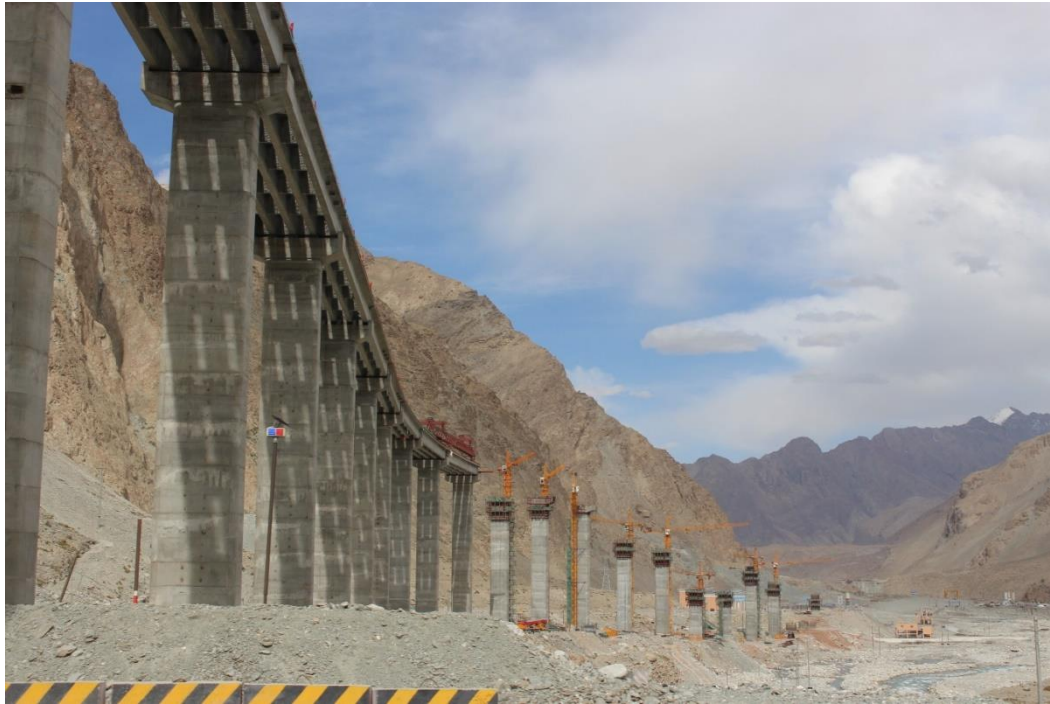
Fig. 6 The advance to the west – Chinese road construction across the Pamir towards Kyrgyzstan
